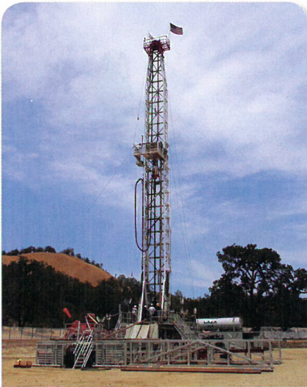
■ Figure 19.26 This drilling rig was used to drill a hole 2.3 km deep in Parkfield, California. Once completed, the hole was rigged with instruments to record data during major and minor tremors. The goal of the project was to better understand how earthquakes work and what triggers them. This information could help scientists predict when earthquakes will occur.
